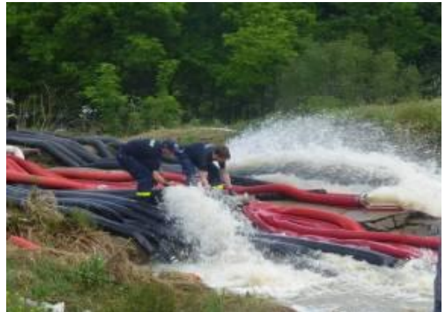
Crews clearing blockages from high capacity pumping hoses in Obrenovac [© Alan Mills MapAction]
